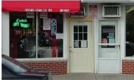
Prohibited: Residential Grade Doors on Commercial Buildings.
